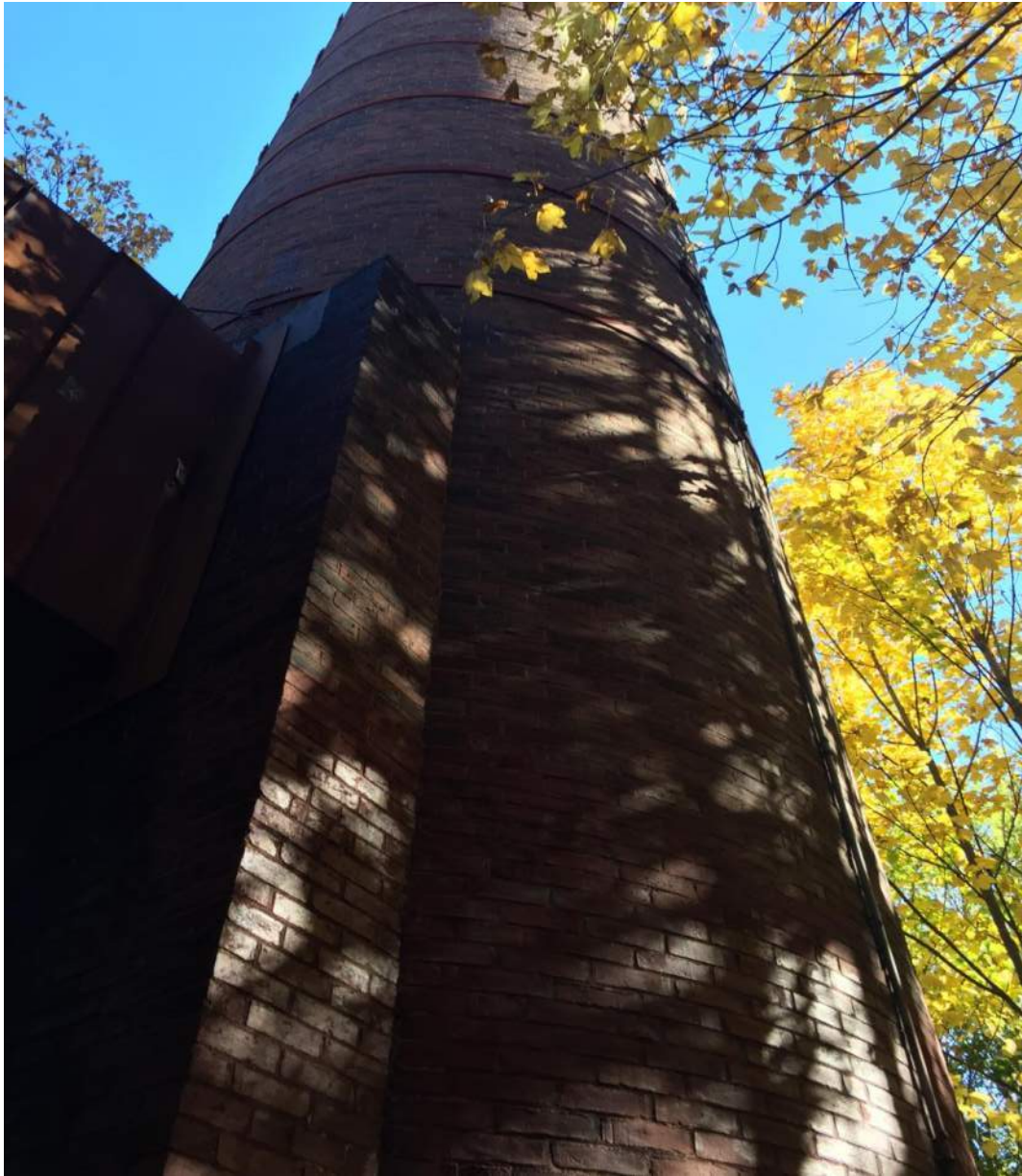
Older Chimney With Possible ACM
