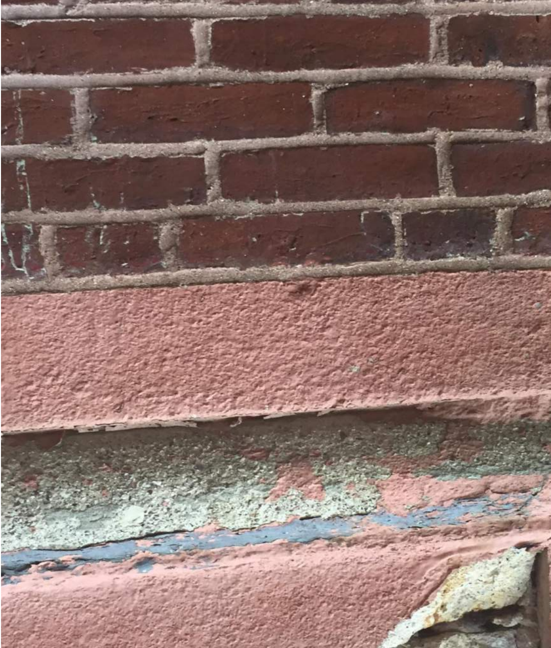
ACM Tar on Coping 1929 D Wing
