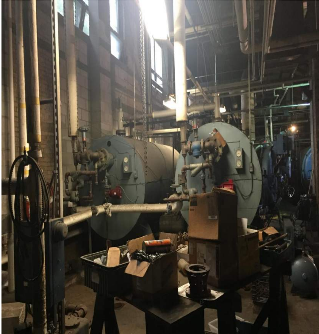
Boiler Room with Fiberglass Pipe Insulation
