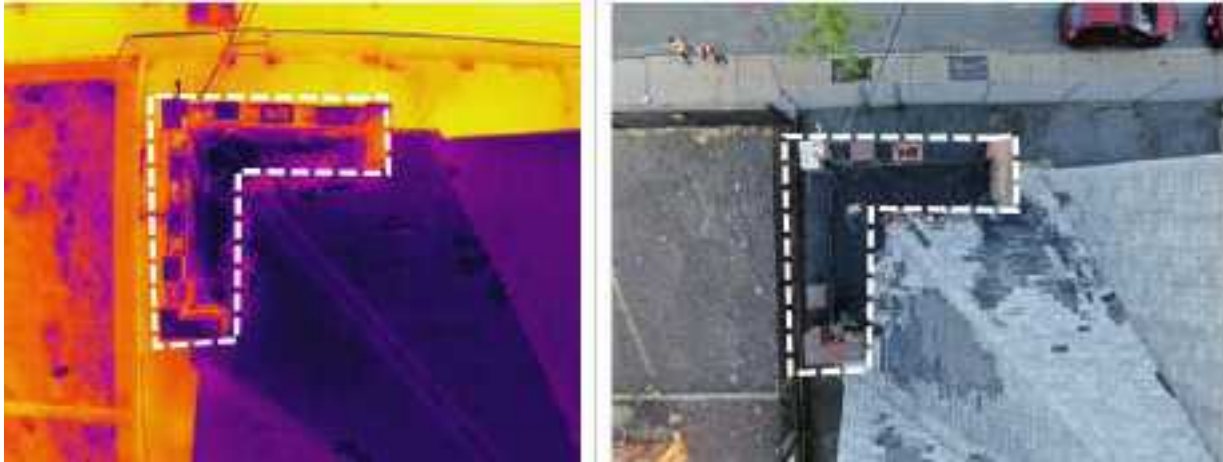
Figure 5. IR image (left) and visual light reference image (right) of thermal anomaly at north corner tower (dashed white area)
