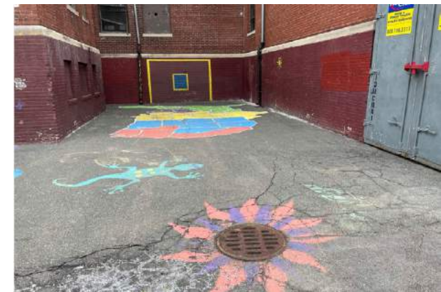
Catch basin in the paved schoolyard at the rear of the building
