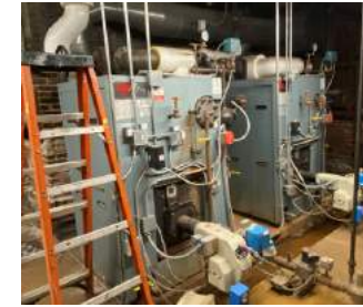
M1, M2. Gas-fired boilers, controls
