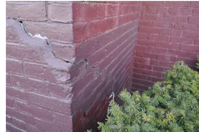
Masonry cracking and displacement, interface of 1901 and 1907 wings
