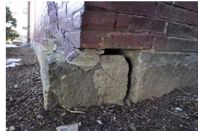
Settlement and displacement of granite foundation units
